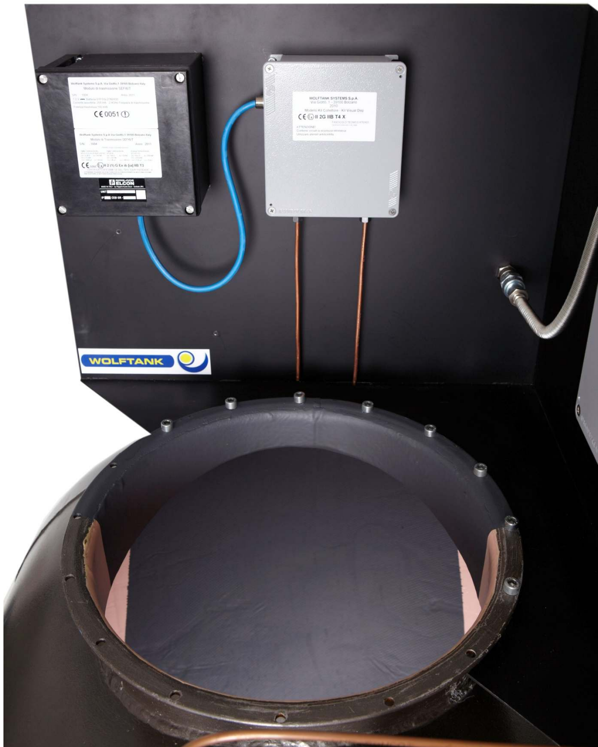
Caption: SEFI 6 monitoring an underground tank transformed by Wolftank.
